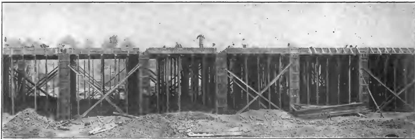
The giant factory plant of the Hudson Motor Car Company at Detroit is rapidly taking shape. The main building, which, when completed, will be one of the model automobile manufacturing plants in the country, is now well above ground and its outlines in reinforced concrete give a good idea of the immensity of the structure.
